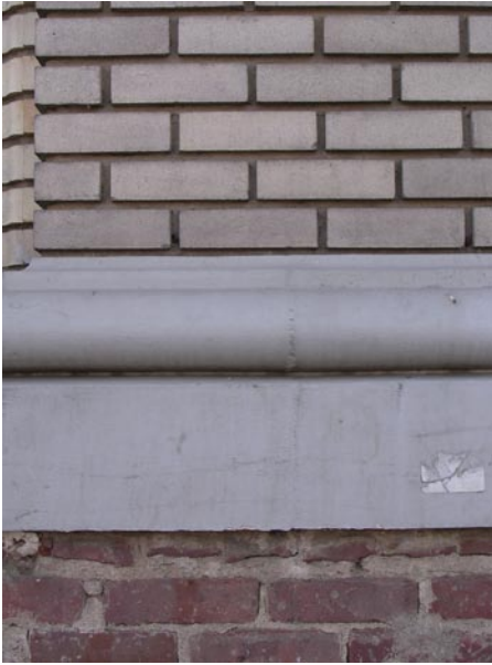
D2, D7 Brick and marble facade on a historic building should be rehabilitated.
