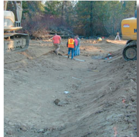
New stream channel will allow steelhead and other fish to access 18 miles of habitat.
