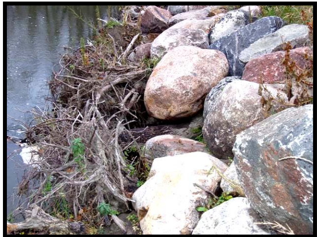
Large rocks used to protect a streambank and to hold rootwads. The river flowed between the rocks, washed the soil out from around the rootwads, and wiped out the entire bank.
