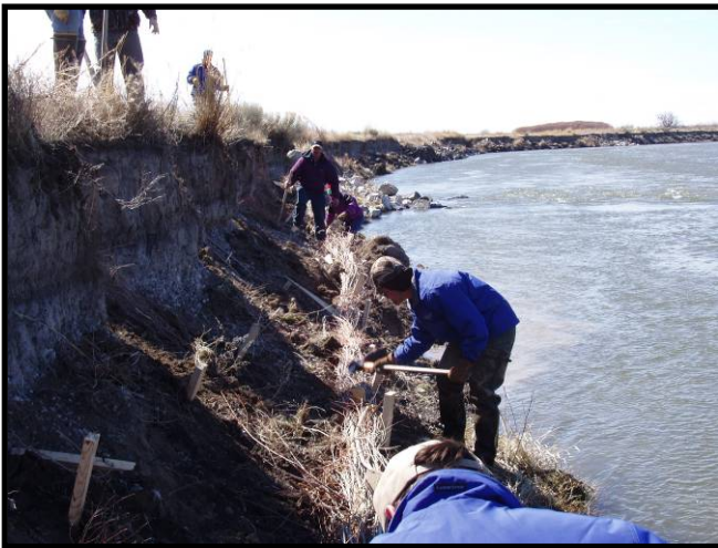
Volunteers install a willow fascine on the bank of the Snake River as part of a training session on the Shoshone Bannock Reservation near Ft. Hall.
