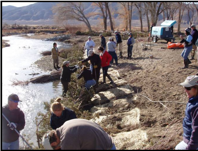
Class installs tree revetments, live cuttings, erosion control fabric, and grass seed at a project on the East Walker River
