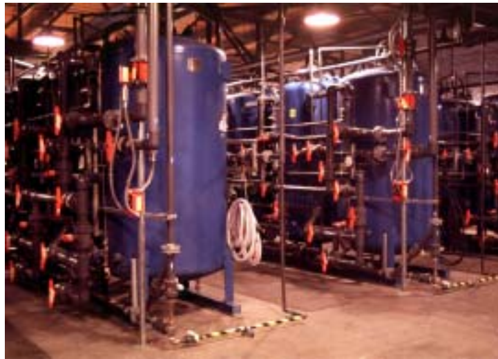
The working parts of a groundwater pump-and-treat system. The groundwater is pumped from the ground and sent through resin-filled columns to remove the contaminants, then injected back into the ground.
