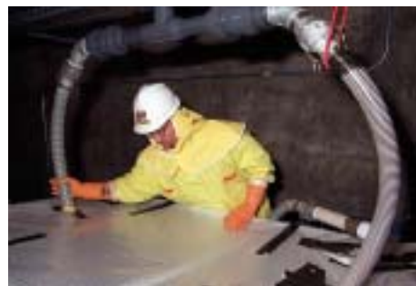
A worker removes spent resin from a pump-and-treat system, then replenishes the system with fresh material. The contaminated resin is safely disposed of in the Environmental Restoration Disposal Facility.
