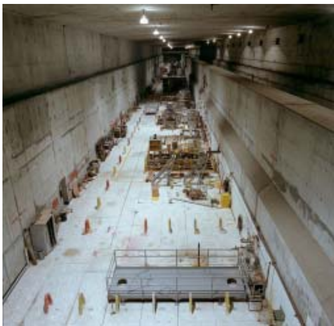
Interior view of the operating deck of U Plant. The feasibility study evaluates the potential for using the canyon buildings as disposal sites for Hanford Site remediation waste.
