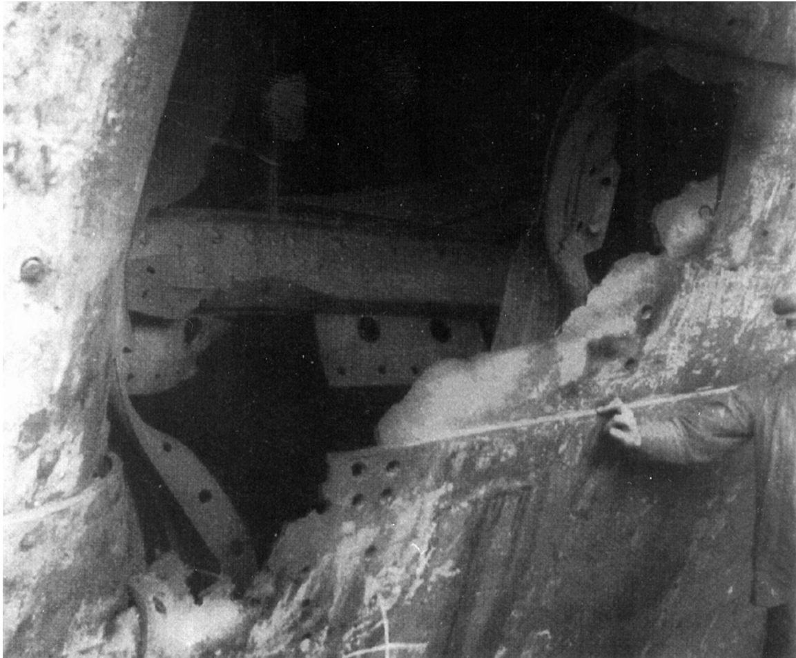
Figure 6: A close-up of the damage to the RMS Olympic due to collision with the HMS Hawke in the Solent in 1911. Note the man for scale. A considerable amount of plasticity in the hull plates is indicated by the bending and twisting seen in the picture. Note missing rivets. Photo from [25].
