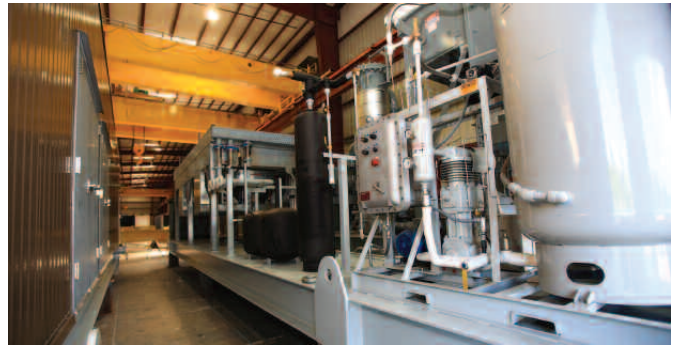
A supporting utility skid for a renewable energy system that contains a methane gas booster compressor, gas conditioning system and heat rejection for the engine PHOTO: STELLAR
