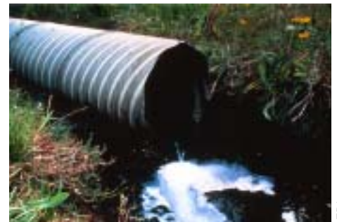
Discharge from pipe
