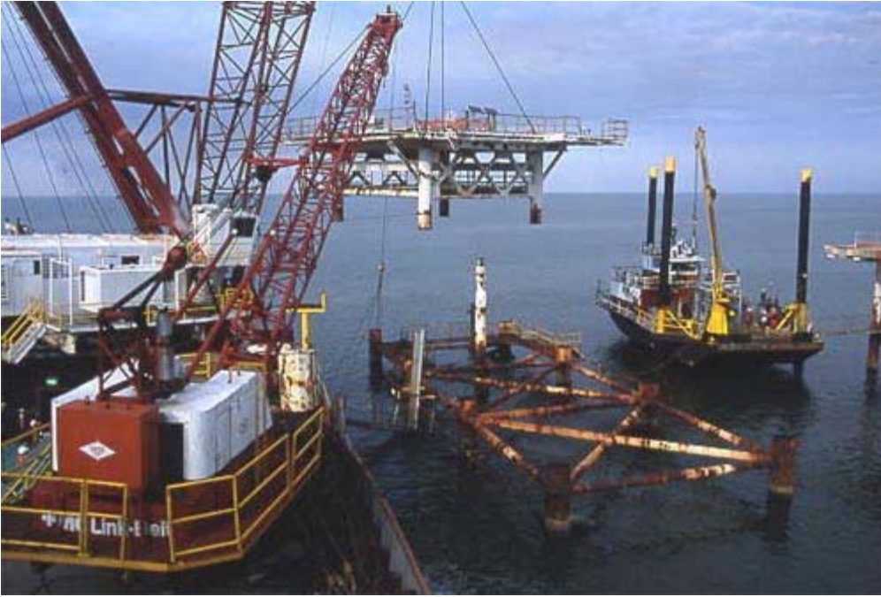
Figure C.4. Derrick Barge Arrives On-Site and Removes the Deck Module (National Marine Fisheries Service – Galveston, 2004).
