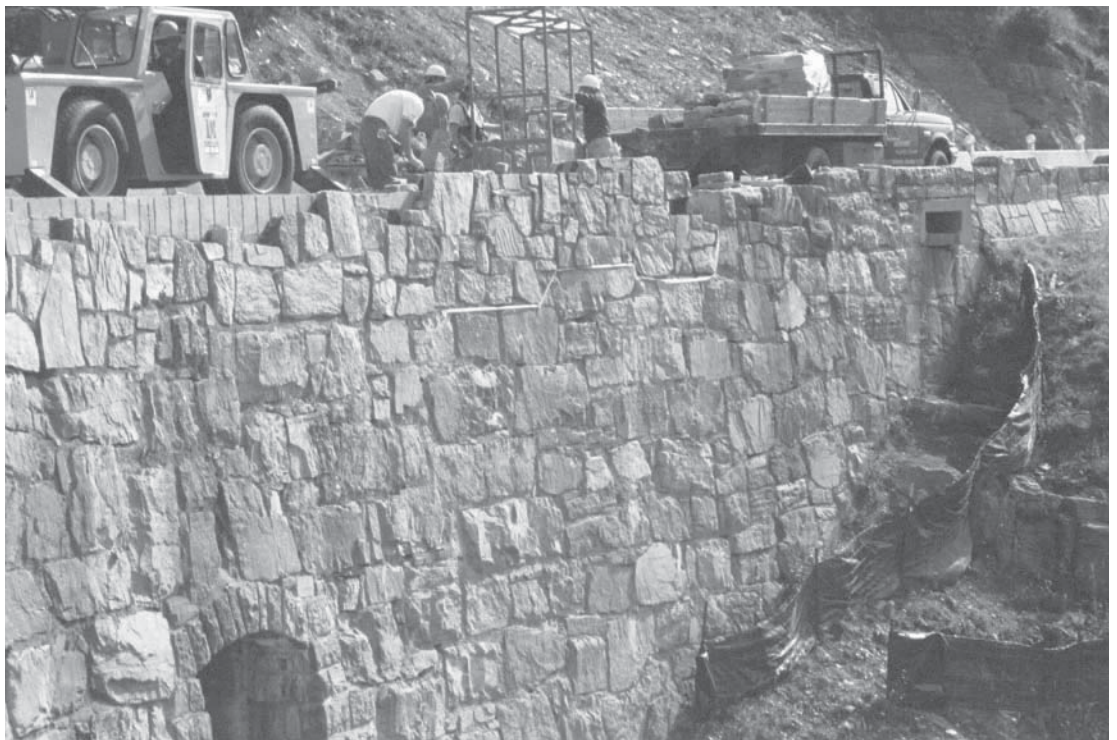
Stone masonry walls, originally constructed in the 1920s, undergo repair and maintenance at Going-to-the-Sun Road, Glacier National Park, Montana.
