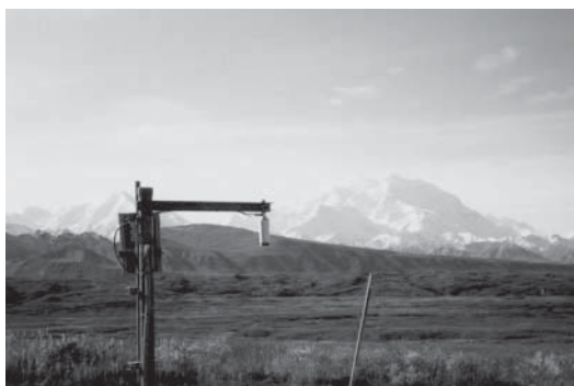
Time domain reflectometry system in Denali National Park, Alaska, provides improved information about winter road conditions.
