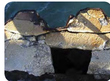
Deteriorated bulkhead on Inner Harbor
