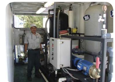
Water treatment facility
