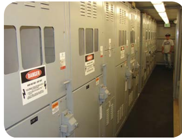
Electrical switch gear
