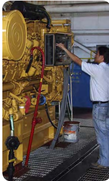
Caterpillar electric generator
