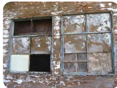
Peeling lead-based paint
