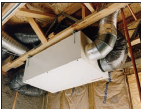
An energy-recovery ventilator ensures good indoor air quality.
