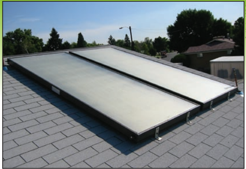
Solar water-heating collectors
