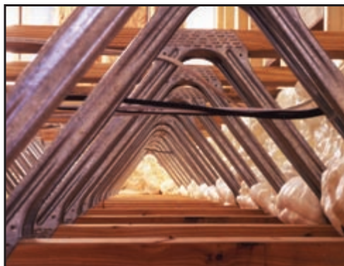
Open web trusses provide space within the building enclosure to run electrical wires and ducts.
