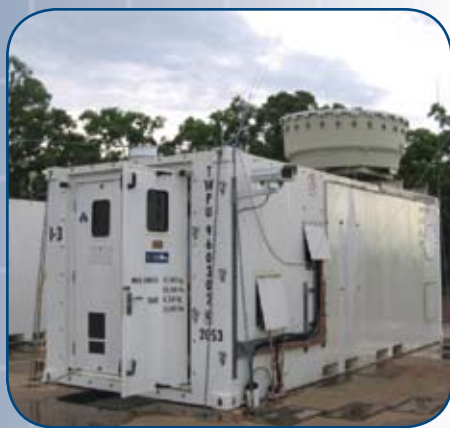
The new processor for the MMCR (antenna shown in upper right of photo) at Darwin collects spectral data in four different modes, resulting in approximately 3.4 gigabytes of signal output per day.
