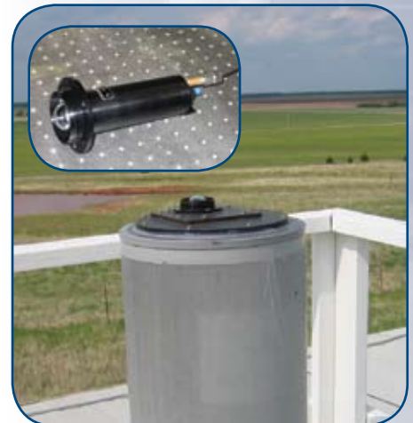
A ceiling port in the SGP Optical Trailer houses the optic element of the SWS, which connects to the spectrometer inside the trailer via fiber optic cable.
