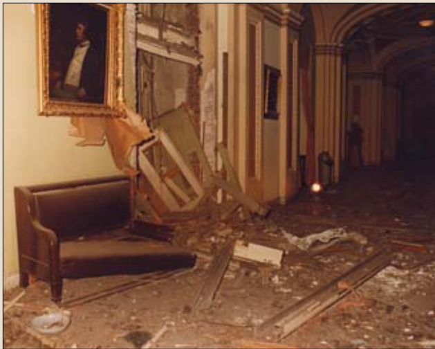
Bomb damage to the second floor of the Capitol, outside the Senate Chamber.
