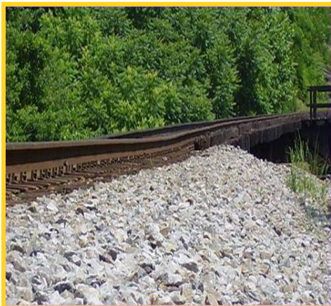
Figure 1. Track settlement at a bridge approach
