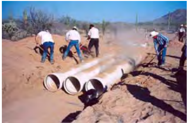
Volunteer work crew installing buried reservoir system at Antelope Tank USFWS Photo
