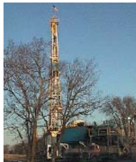
Photo courtesy of GTI and the GTI Catoosa™ Test Facility.
