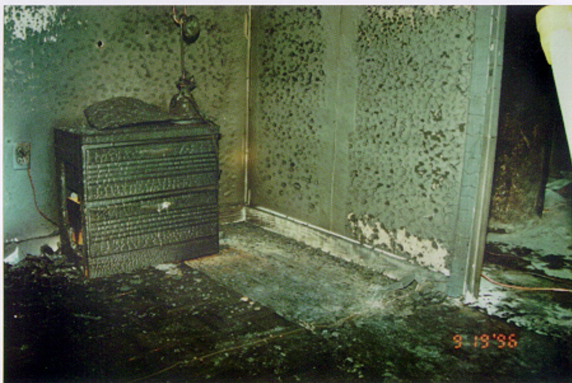
FIGURE 58. Photograph showing damage to the side of the nightstand, Experiment 3.
