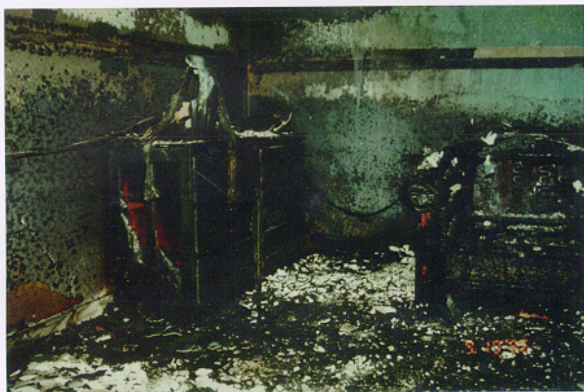
FIGURE 56. Photograph showing damage to the side of the dresser. Experiment 3.
