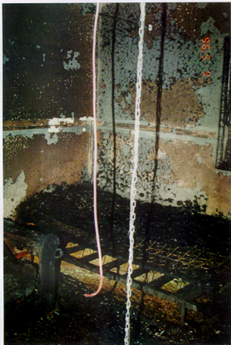
FIGURE 38. Photograph of the condition of the bed and the protected floor area below. Experiment 1.
