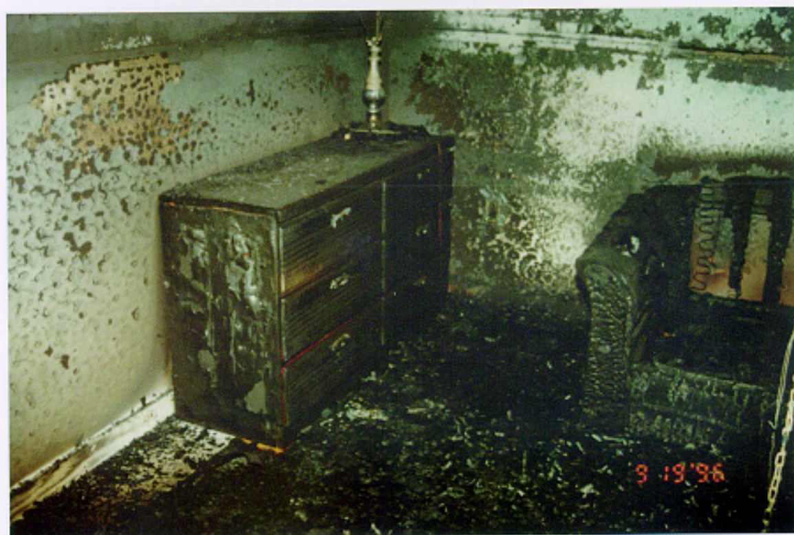
FIGURE 57. Photograph showing damage to the side of the dresser. Experiment 4.
