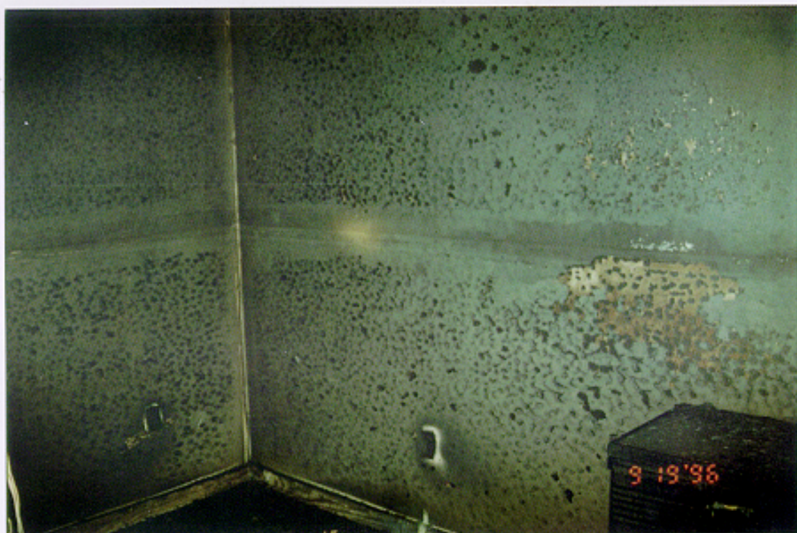
FIGURE 61. Photograph of the wall behind the door of the room, which was consumed by fire. Experiment 4.
