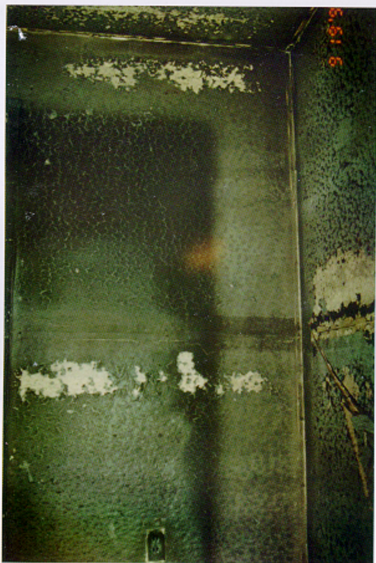
FIGURE 60. Photograph of the wall behind the door of the room, which was consumed by fire. Experiment 3.
