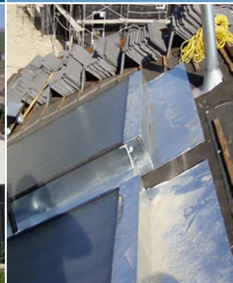
(left, right) ICS mounted directly on roof deck and integrated with mission and cement tile systems. The photos were taken at a development in Thousand Oaks, California, in 2002. Photos courtesy of John Harrison of the SRCC and FSEC.
