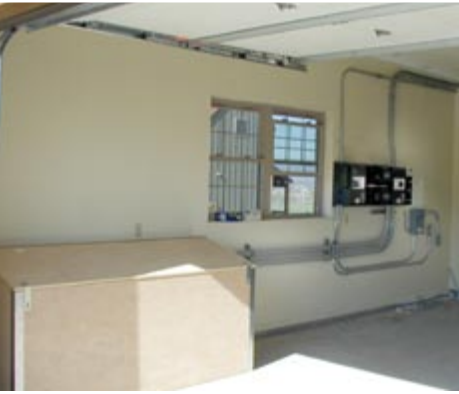
Residential inverter with backup batteries stored inside the box. Photo courtesy of Leif Juell, Alternative Power Enterprises, Inc.
