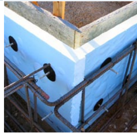
Clarum is building four zero energy research homes at Borrego Springs, California. Polystyrene slab edge insulation helps to carefully control heat gains and losses. Photos courtesy of Clarum Homes.
