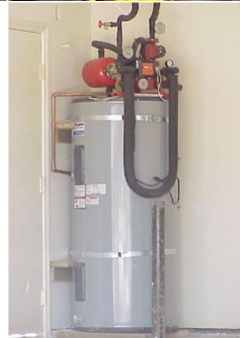
(left) Rough-in plumbing for a solar thermal system. Photo courtesy of Heliodyne.
