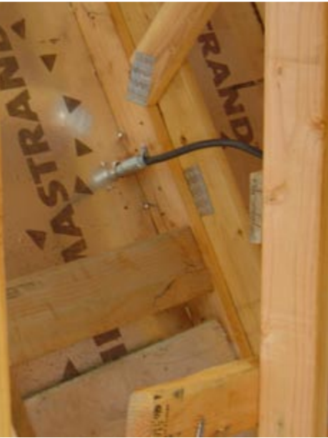
(left) Added lumber makes PV module installation easier. The added cross piece in this photo is located just below the wire penetration.
