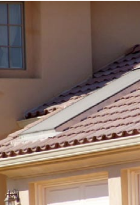
Although visible, solar thermal systems that sit above the roof have low silhouettes and resemble skylights.
