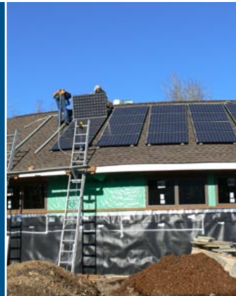
Contractors install PV panels on the curved roof of this custom zero energy home near Olympia, Washington.
