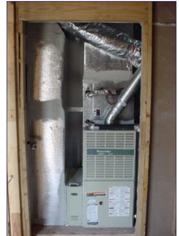
A fresh air intake duct with a Constant Airflow Regulator runs from the outside to the return plenum. The furnace operates continuously on low speed to provide whole-house ventilation.
