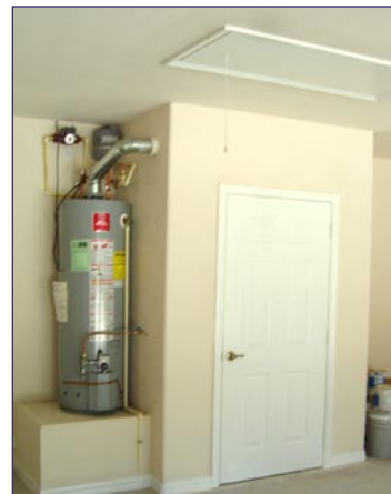
FIGURE 17: Air Handler in Conditioned Space
