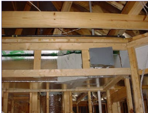
The final duct installation incorporated a horizontal duct board trunk in the bulkhead with flex duct runs perpendicular to this main trunk.
