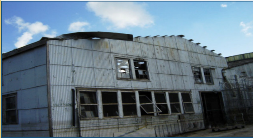
BEFORE: This warehouse once served as an inmate training facility and storage area for materials and supplies for the Orleans Sheriff's Office. Source: FEMA Photos
