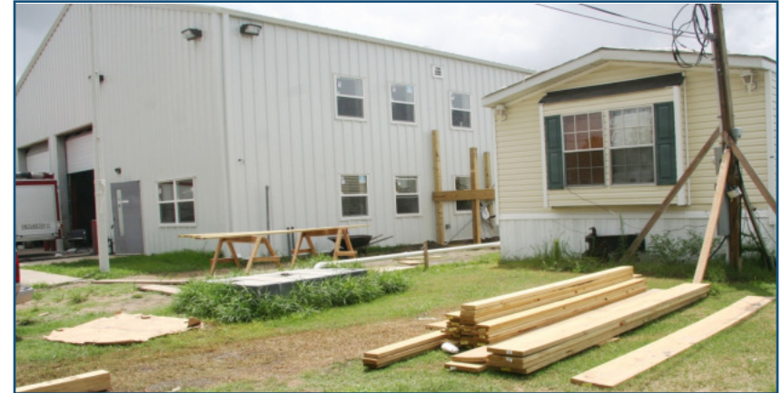
AFTER: Renovations at Station 1 in Arabi are near completion even as the firefighters continue to use the temporary trailer that sits next to the building. Source: FEMA Photos
