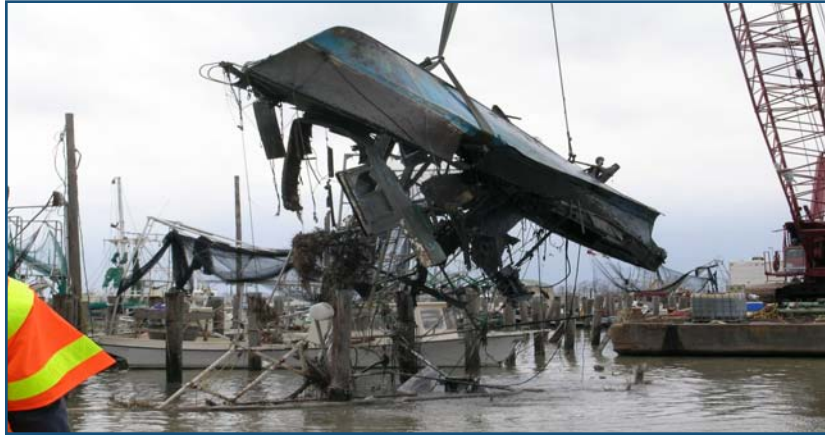
BEFORE: Teams of local, state and federal officials remove debris from Louisiana's waterways, including boats and other marine vessels. Source: U.S. Coast Guard
