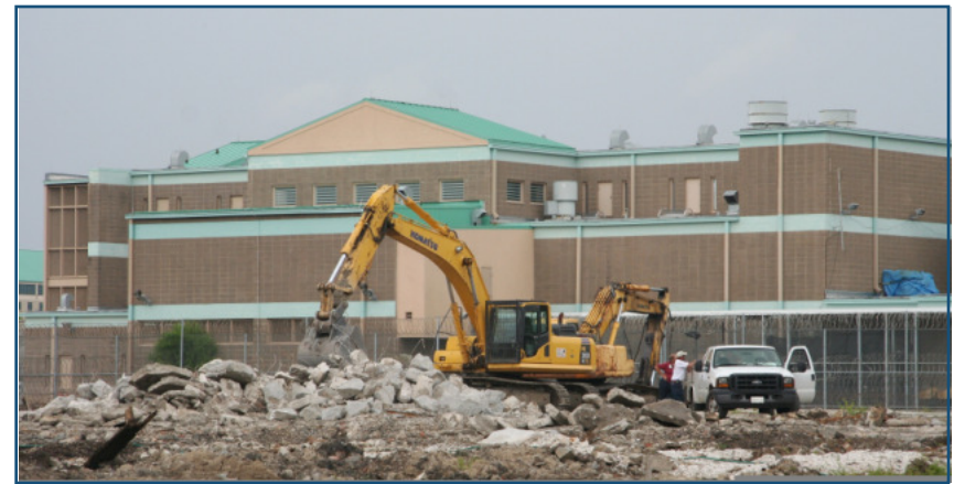
AFTER: The remains of the old warehouse site were removed in May 2008 in preparation for the construction of a new main kitchen for the sheriff's complex. Source: FEMA Photos
