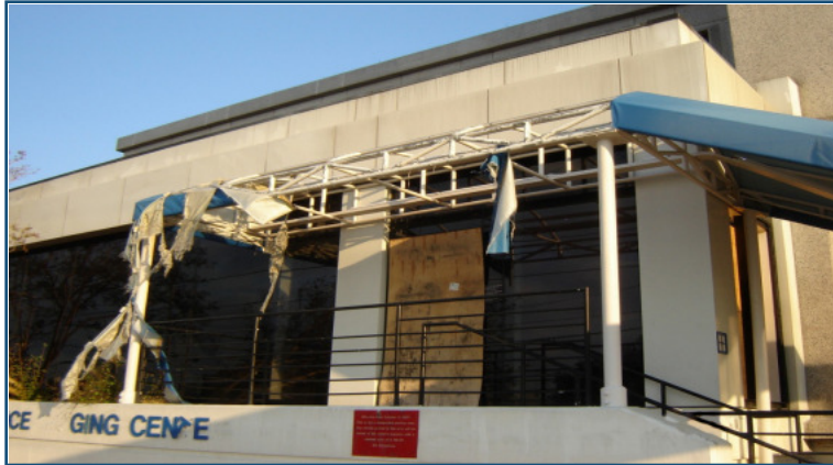
BEFORE: Located in New Orleans' Central Business District near the Louisiana Superdome, many of LSU's medical buildings were severely damaged by floodwaters. Source: FEMA Photos
