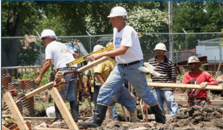
BEFORE: Construction has already begun on the expansion across from Chalmette High School as these workers install pilings and a foundation. Source: FEMA Photos
