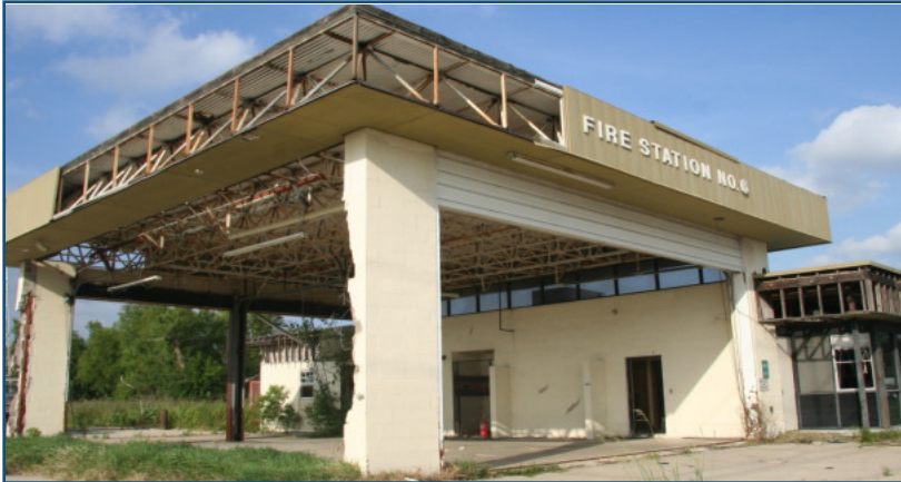
BEFORE: This station, #6 in Meraux, La. is an example of the destruction sustained by St. Bernard Parish's fire department. Station 6 is in the design phase for renovations and expected to be completed by 2009. Source: FEMA Photos
