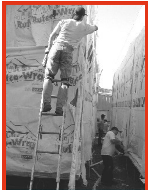
Home Sweet Energy-Efficient Home: The set-up crew assembles a home made from foam core panels that could reduce heating and cooling costs by as much as 50%.
