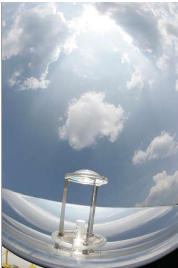
The collector for the hybrid solar lighting system, mounted atop the roof of a building, tracks and captures the sun's rays to light the rooms beneath.
