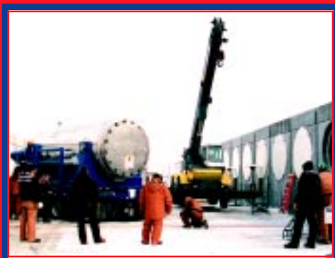
Trailer carrying a shipping cask from Three Mile Island is carefully aligned to push the shielded canister into a spent fuel storage module at INEEL's spent fuel storage installation.
