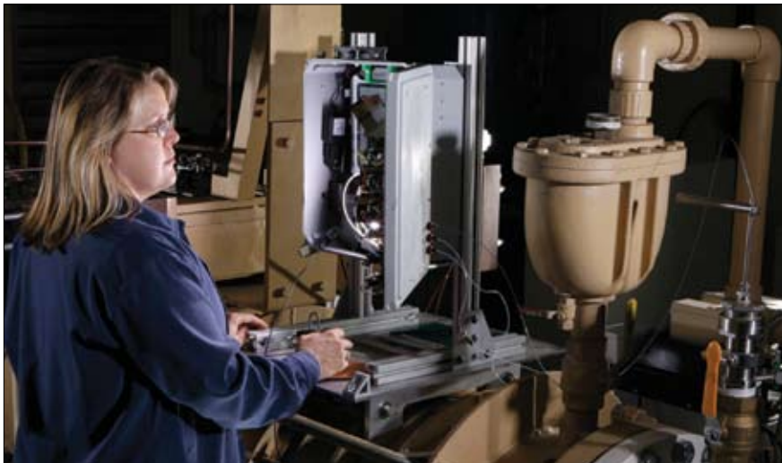
Victoria VanderNoot, an analytical chemist at Sandia, observes operational data displayed by the lab's unattended water sensor (UWS), shown here at a large water utility in San Francisco's Bay area. The UWS has undergone testing at the utility site for more than a year and is now deployed at a municipal water station in Arizona, where operating parameters continue to be fine-tuned.
