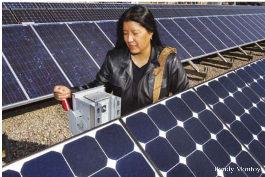
Debby Tewa with photovoltaic units at Sandia. She is helping Native Americans in remote areas learn how to maintain PV units deployed via DOE grant money.
