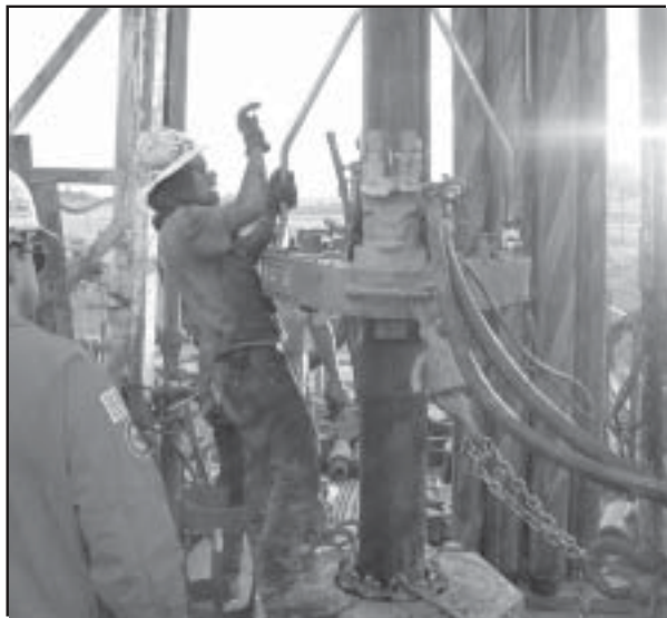
Workers run casing into the well after a ProDril test. ProDril Services, Inc. injects steel shot into drilling mud to increase the penetration rate of the drill bit through rock. The process will reduce the time and cost required to drill deep, hard rock formations.
