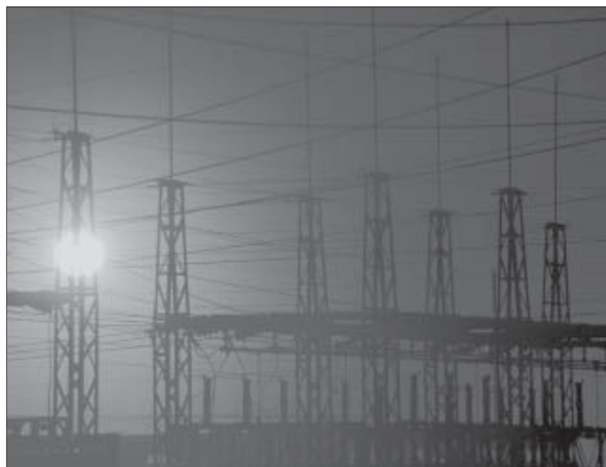
The Risk Assessment Methodology provides a formal process for evaluating and improving the security of critical elements of the U.S. infrastructure.
