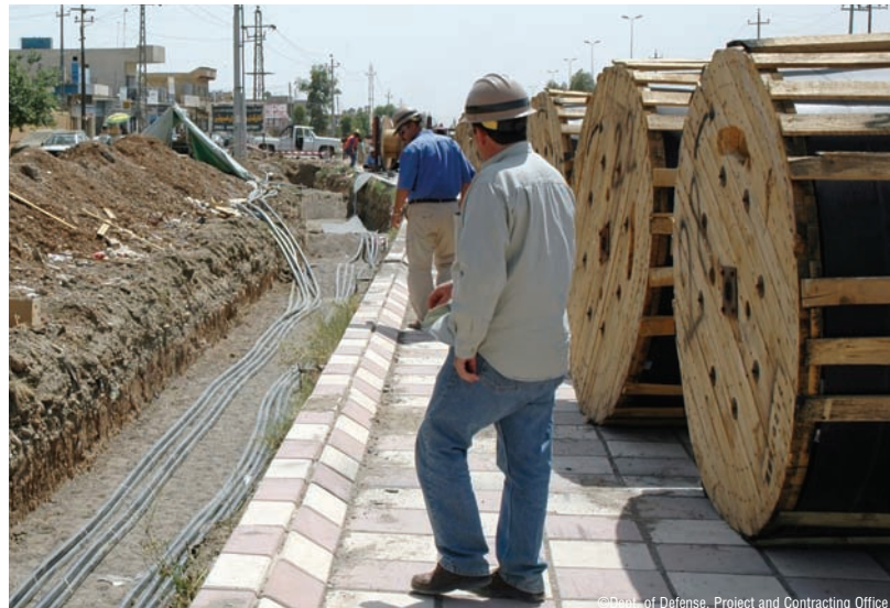
Iraqi workers on an IRRF project inspect recently dug cable trenches to ensure underground power cables have been laid correctly. Improved electrical services for local Iraqi homes and businesses will decrease dependency on neighborhood generators and provide a more continuous supply of power for local residents.
