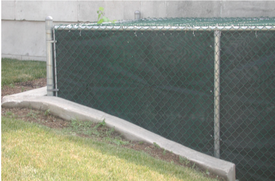
Meter set assembly protected by a chain link fence, both top and sides, with the posts anchored to a concrete wall.
