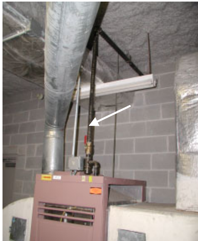
Fuel Line Providing Gas to Space-heating Furnace
