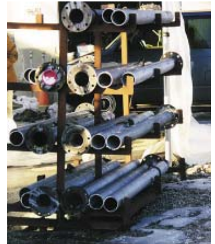
Disassembled Piping Awaiting Decontamination in Hot-Gas System
