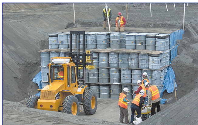
Hanford Site: Workers are removing drums containing suspect transuranic waste from a retrieval trench in the middle of the site. By mid-March 2004, more than 1,600 drums had been retrieved.
