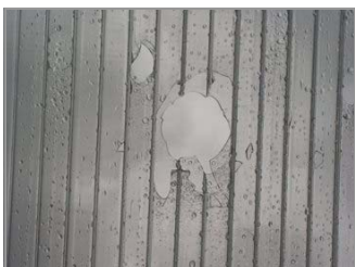
Hole in main greenhouse side wall
