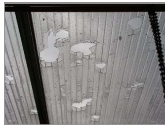
Main greenhouse roof damage close-up
