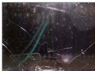
Broken window to lathhouse
