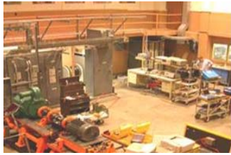
Motor Systems Resource Facility
