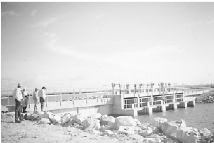
Water control structure at Salt Bayou, McFadden Wetlands, TX.
