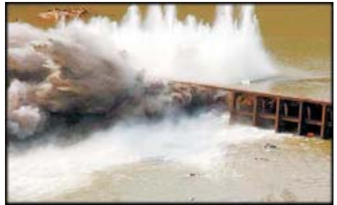
Army and Air Force personnel used explosives to demolish a 100-foot section of the Embry dam, providing a valuable training opportunity for our soldiers.
