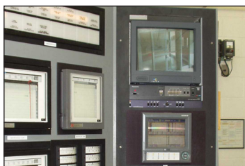
Digital recorder upgrades
