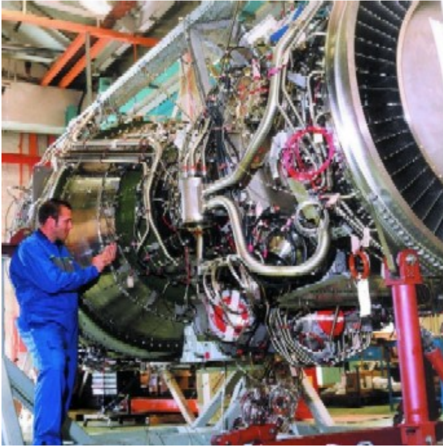
Figure B-2: Close up of Piping to Dry Low NOx Combustor System
