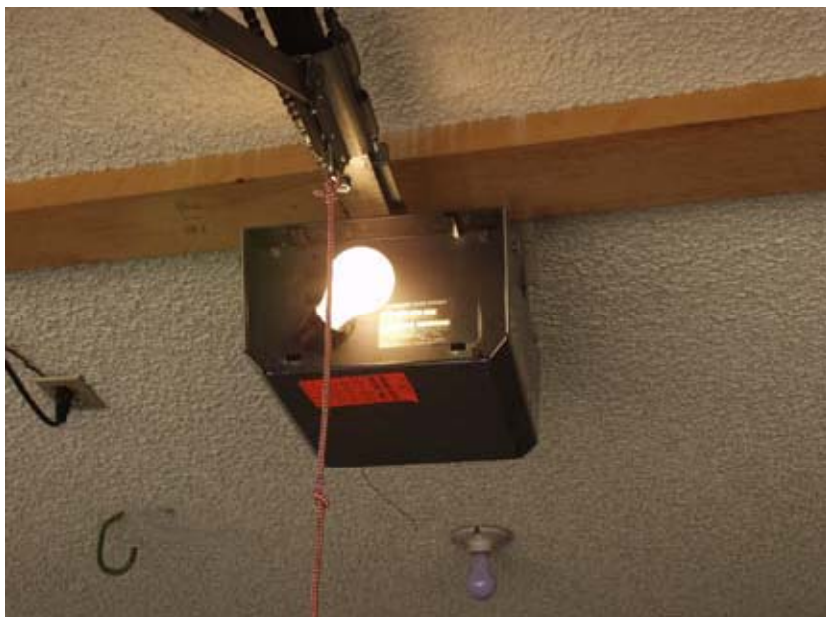
Garage Door Opener
