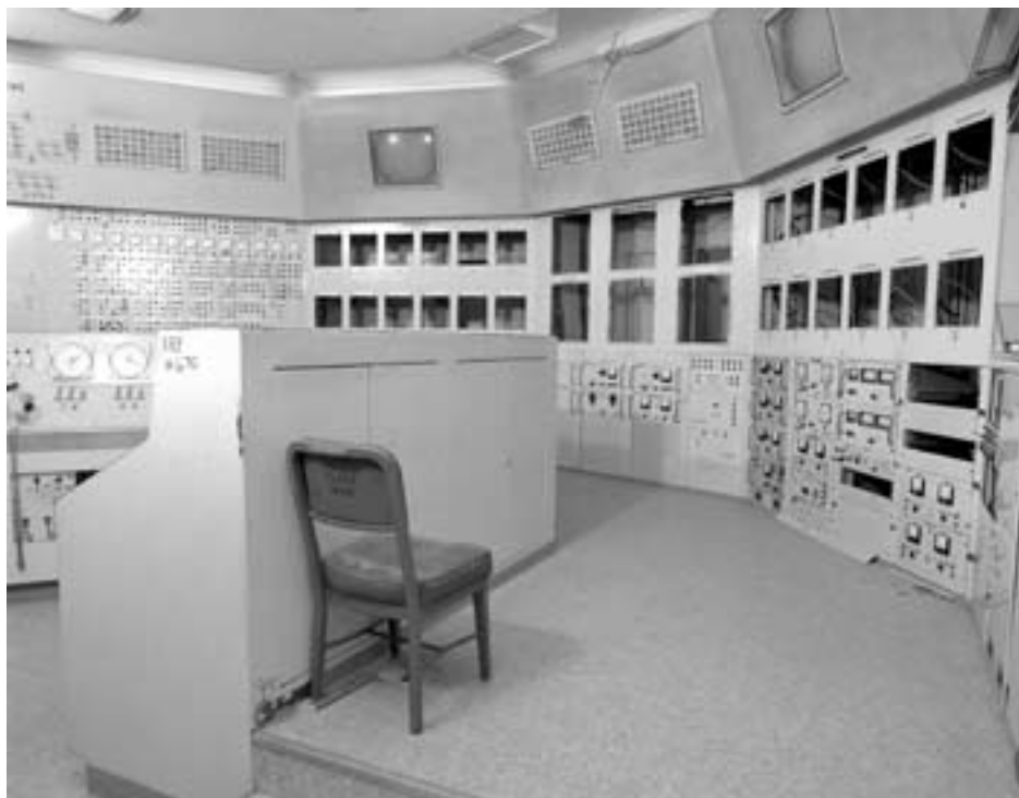
The control room in 2001 with holes in the walls showing where instrumentation had been “cannibalized” for use elsewhere. (NASA C-2001-01221)
