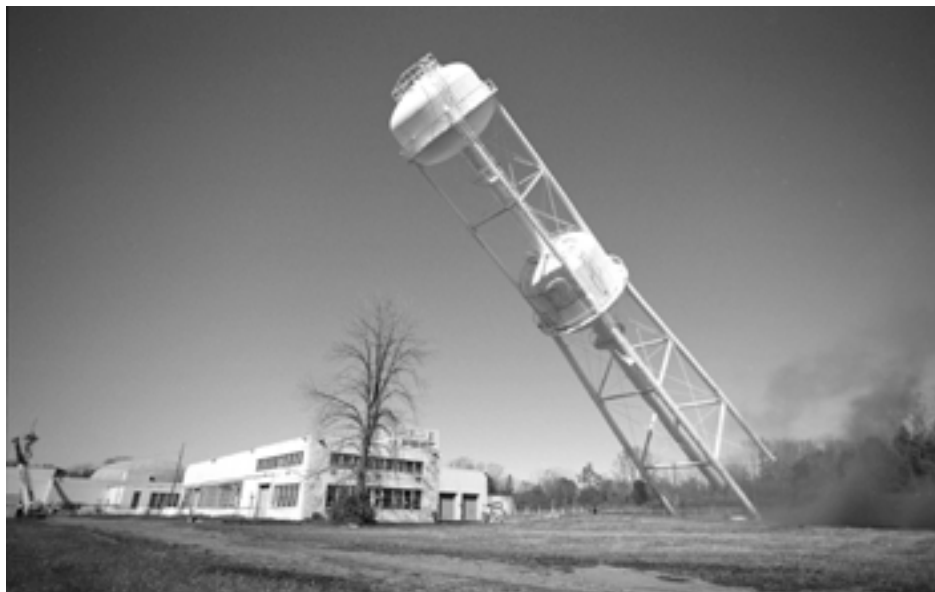
One of the most dramatic moments of the decommissioning process was the demolition of the water tower. (NASA C-2004-744)
