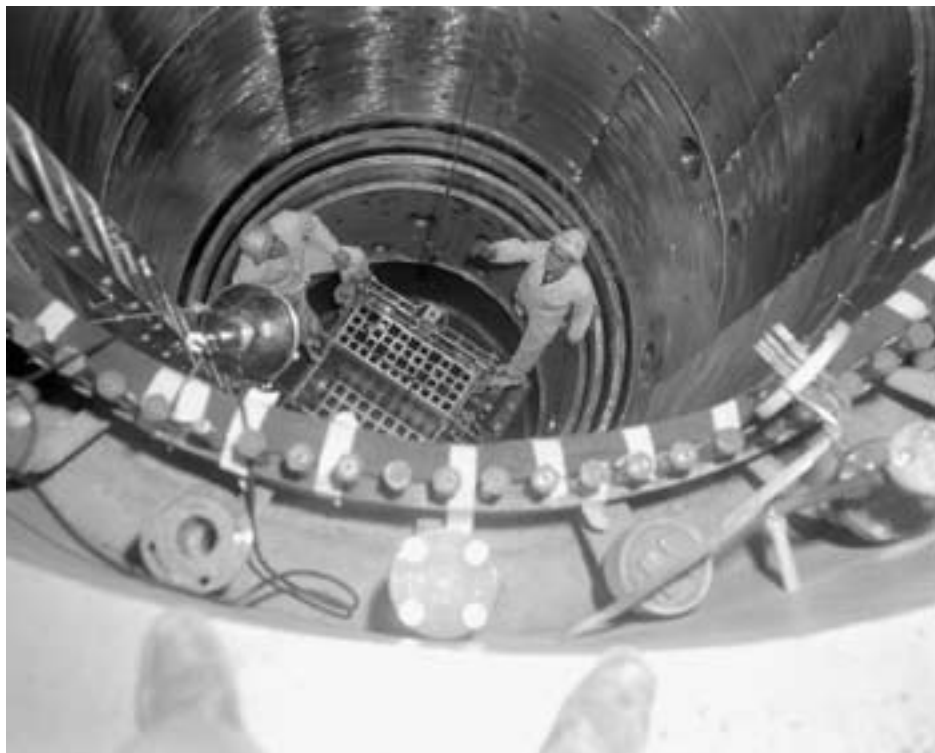
Engineers working on the installation of the reactor core where experiments would be inserted. (NASA 1960_55018)
