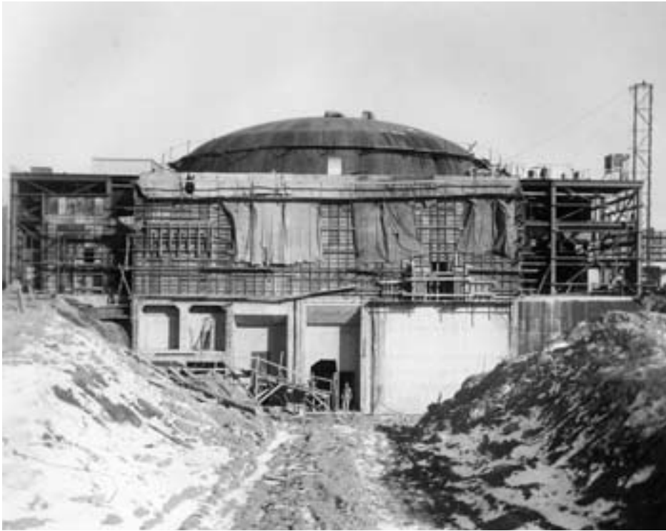
Side view of the construction of the containment vessel and main reactor area. (NASA 2005-1203)
