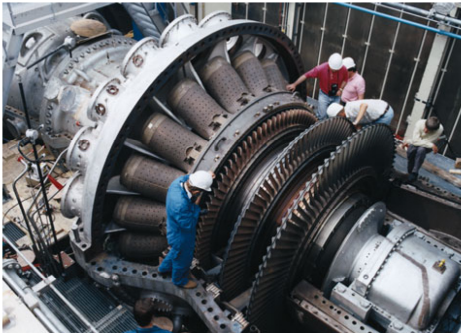
Figure 7: Turbine rotor showing the turbine blade disk and blades. (Image: Courtesy of GE Global Research Center)
