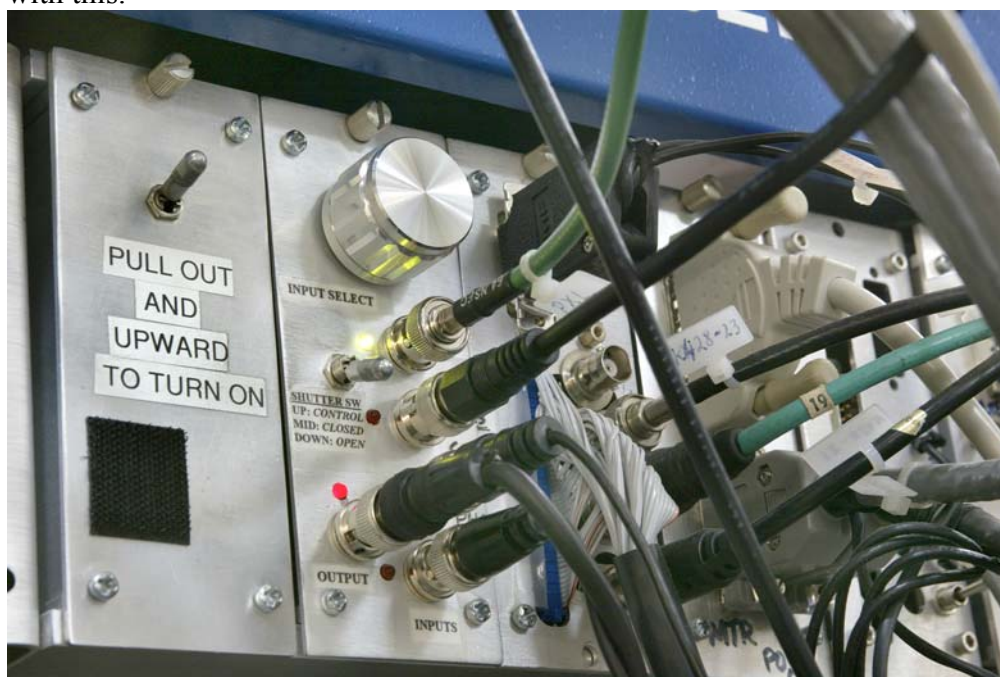
Shutter Switch at BL 12 (left of green BNC cable, below round knob)
