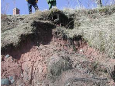
Eroded slope, subsurface seepage on Outer Island
