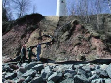
New rock revetment, drain tile from top of slope cutoff trench, on Outer Island
