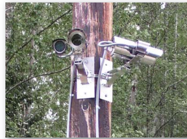
VPED camera installation at a road junction.
