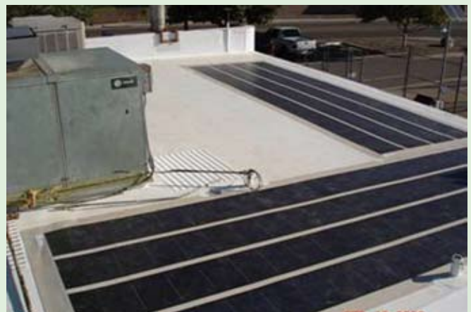
The New Photovoltaic Roof on Building 833
