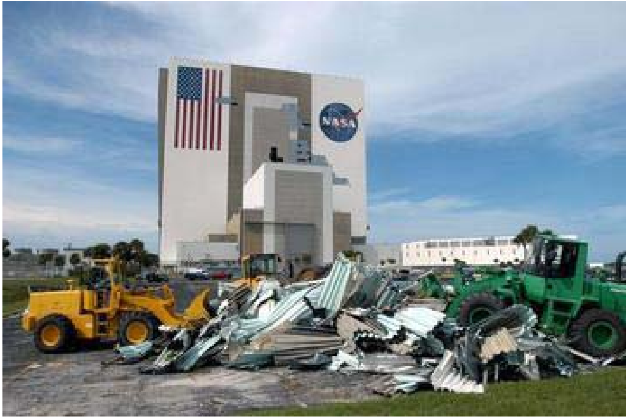
Vehicle Assembly Building (VAB) (K6-0848) – debris pile from exterior panels
