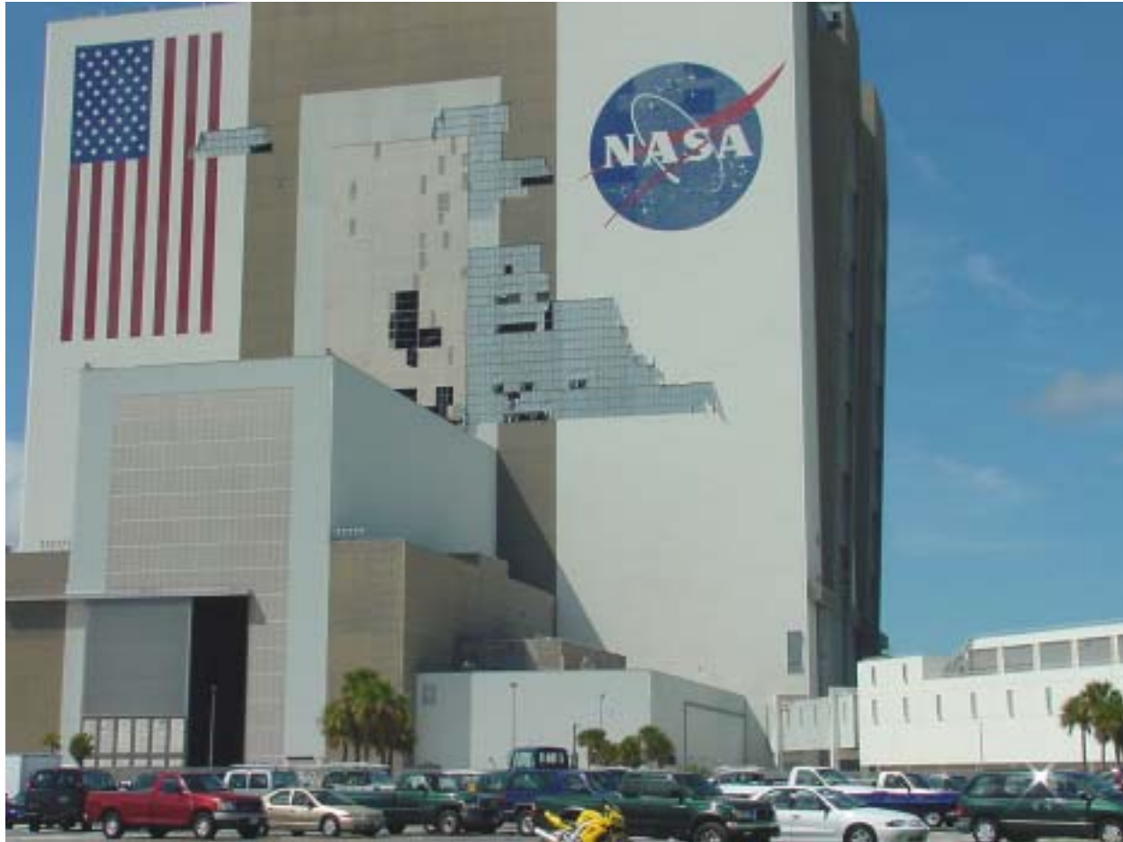
Vehicle Assembly Building (VAB) (K6-0848) – exterior panel damage (south side)
