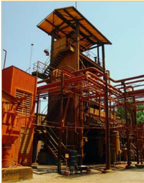
Part of the World War II carbonyl iron plant in the Carbonyl Iron Unit Historic District at Redstone Arsenal. This is one of only three known active carbonyl iron plants in the world. The district has undergone very little modification since it first began production in 1943.
