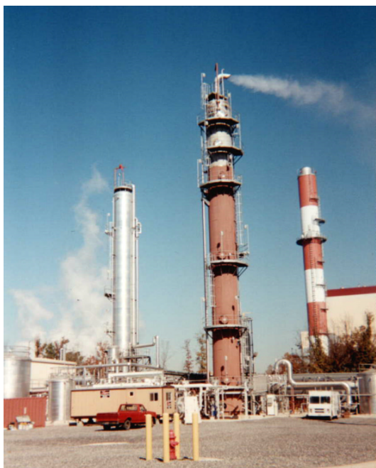
Figure 3. CO 2 capture plant at Warrior Run power station (courtesy AES)
