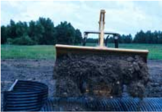
Lofton water control structure Tensas River National Wildlife Refuge
